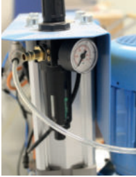
Fig. 4: Pneumatics servicing unit
